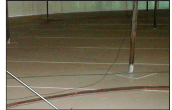
Final inspection of the ARC lining to ensure a continuous pinhole free protective lining
